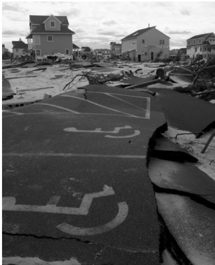
Accessible parking spaces destroyed by Sandy
